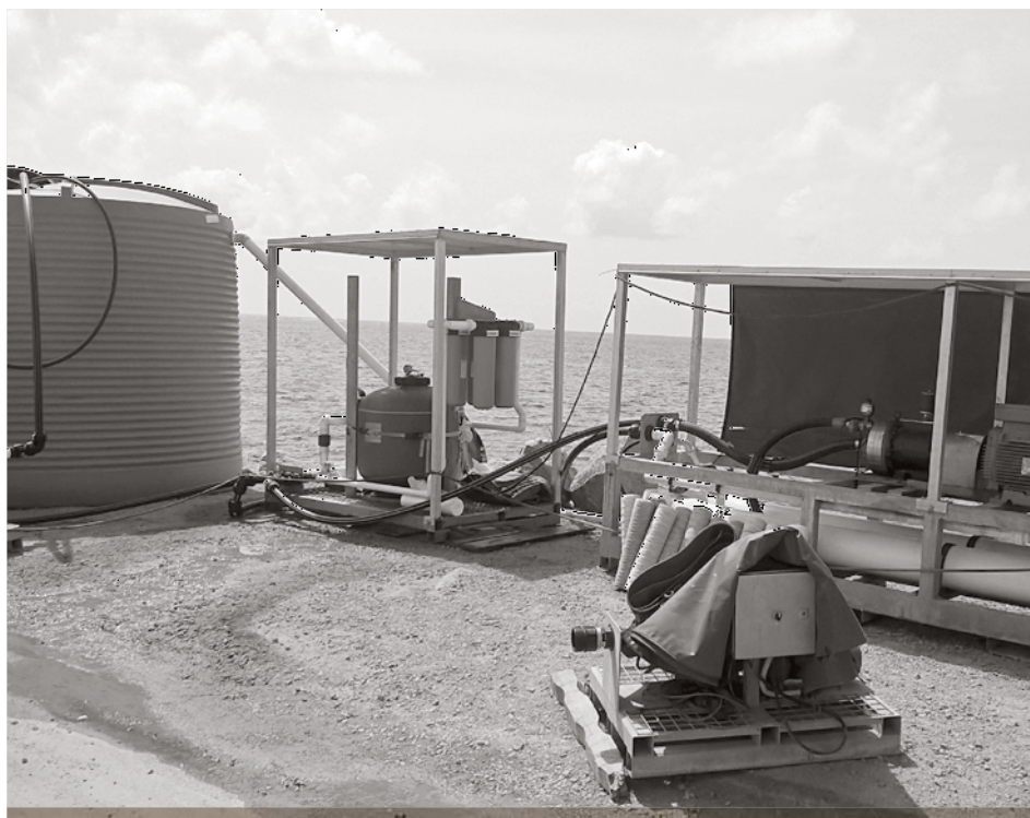
MOBILE DESALINATION UNIT.
